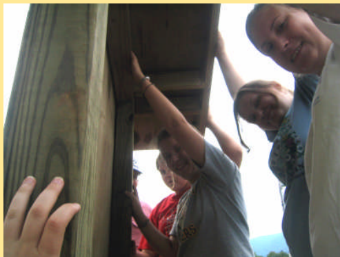
2006 Team Members erect the outdoor prayer shrine, which they designed and constructed.
